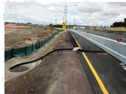
Figure 18: Hotmix bund diverting the motorway runoff to the catchpit
